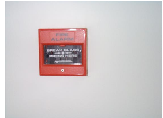
Break glass fire alarm
